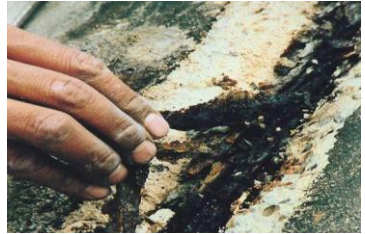
Internal damage at Grace Cathedral due to their prior failure to waterproof their concrete walls
